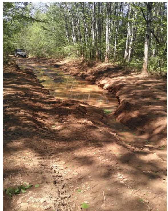
Trail Washout in Lynne Needing Repair
