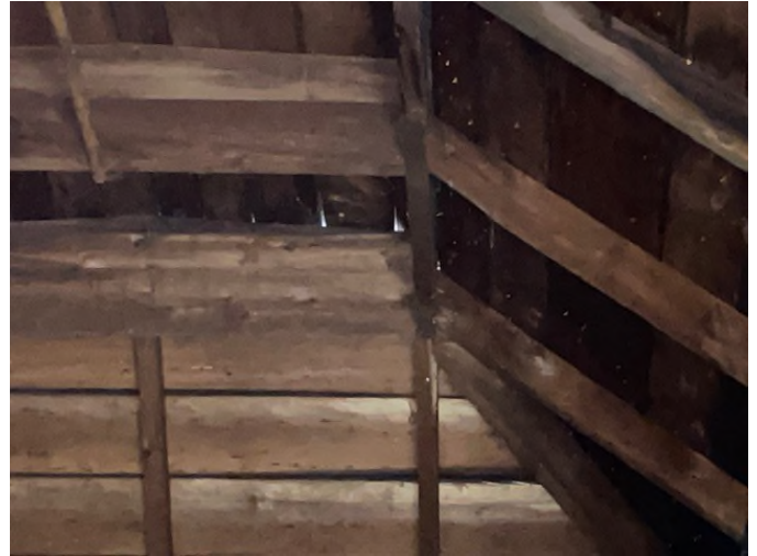
Holes in garage roof
