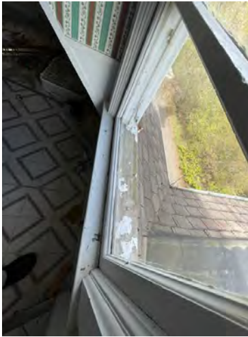
Exterior window - missing paint
