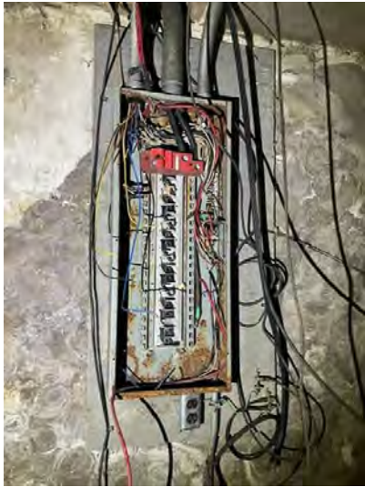
Usable part of service panel removed - Note rust from high humidity
