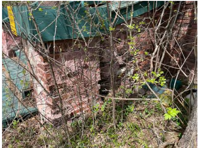
Front porch deterioration
