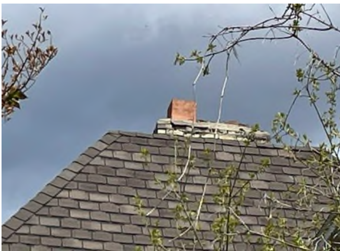
Deteriorated chimney, part missing
