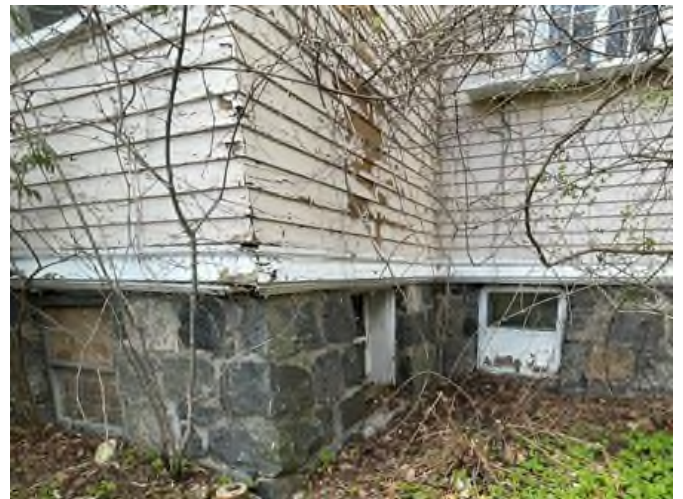
Deteriorated siding and band board
