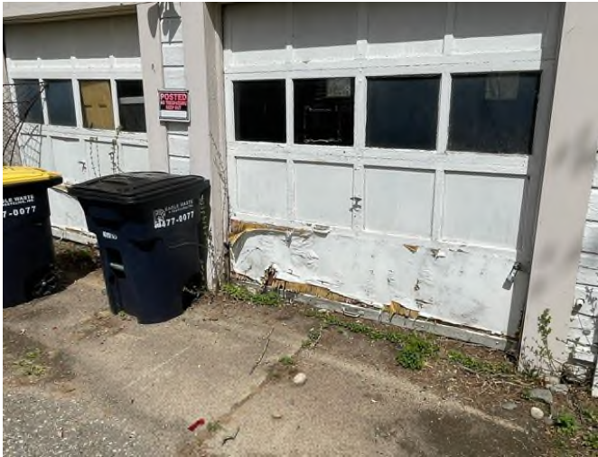
Severe garage damage
