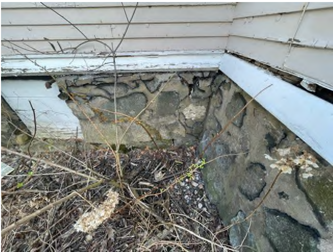
Foundation settlement & damaged band board
