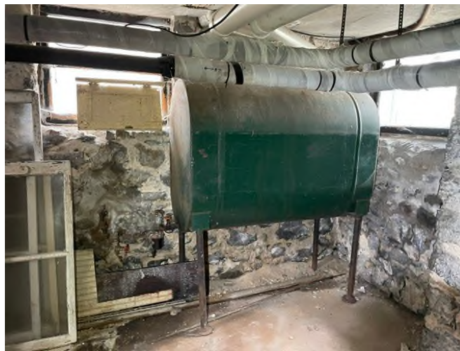
Old fuel oil tank in basement
