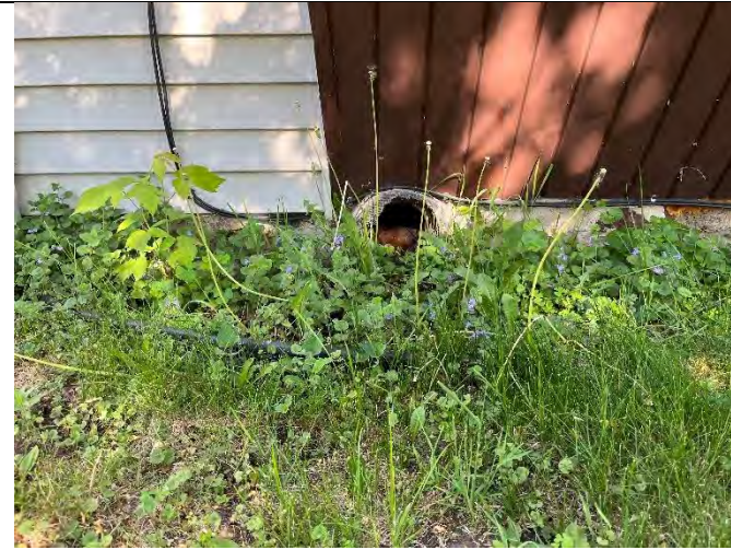
Drain coming out of front of house.
