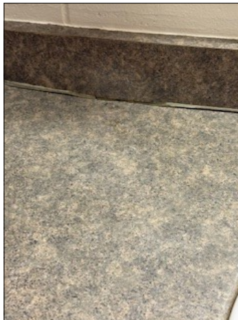
Countertop in one of the basement bathrooms with missing caulk.
