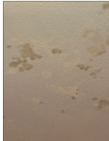
Ceiling in a shower
