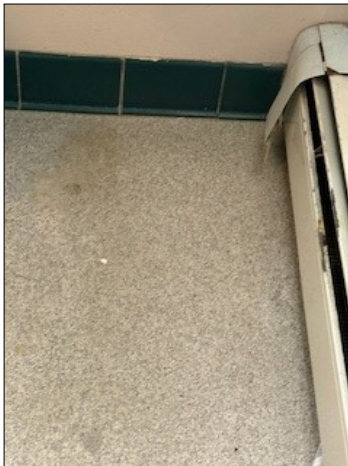
Floor boards (that's what they're called, right?) They have seen better days.
