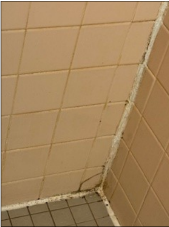
Bruce said the mold keeps coming back where new caulk was put in. They did a really bad job caulking.
