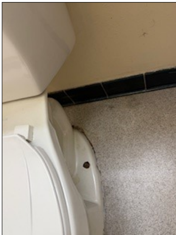
Caulking around the toilet is cracked. This would probably be fixed when new flooring is put in but if not the caulk should be replaced.
