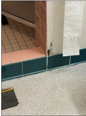
Hole in the wall. I think I only saw this in one bathroom. A number of others had peeling paint (see picture below) but I didn't see any other holes.
