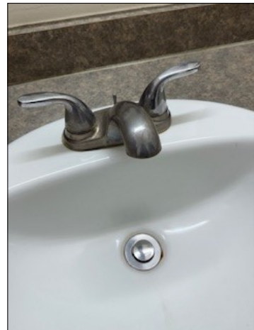
Faucet. They are just looking very worn and seems like it could be a relatively "cheap" fix.
