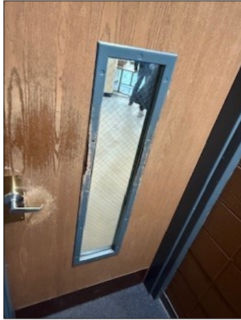
Door leading to the basement. Many of the doors looked like this.
